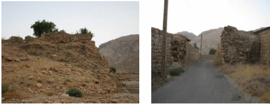
Fig 9: Entrance and view of fence of Amir Seif Castle at northern side (Author: June 2013)
